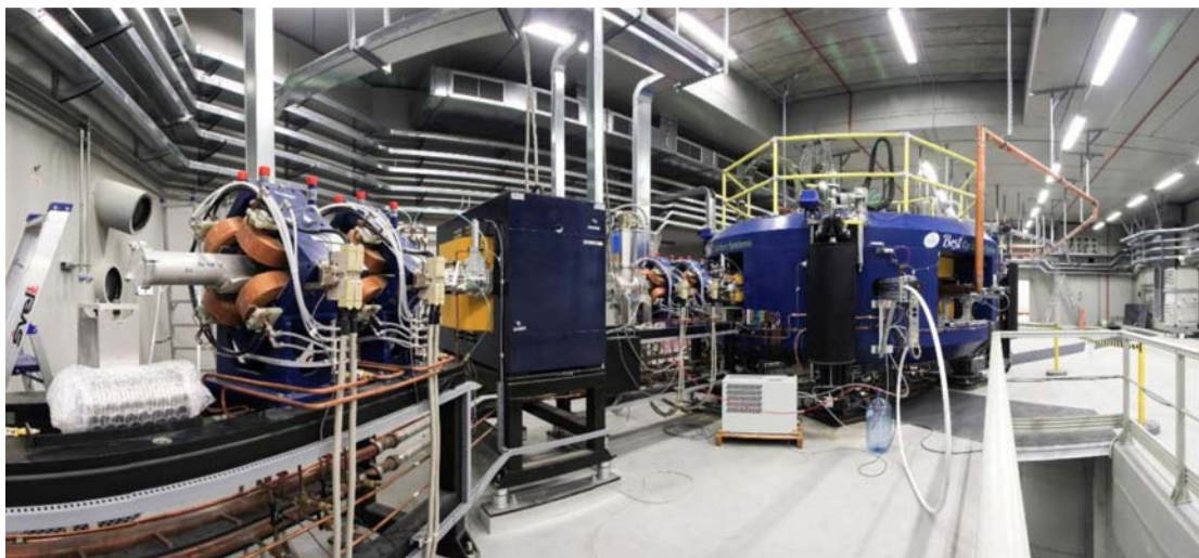
Figure 2. The B70 cyclotron installed at LNL.
